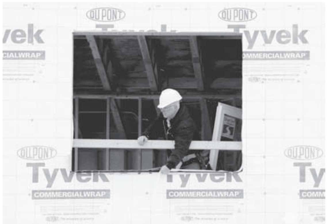
A builder works on a home under construction in northwest Chicago. U.S. homebuilders' confidence in the housing market rose modestly in April but remained at low levels for the third straight month, constrained by tight credit for home buyers and a shortage of workers and available land, according to a National Association of Home Builders report released Tuesday, April 15, 2014. (AP Photo/Nam Y. Huh)
